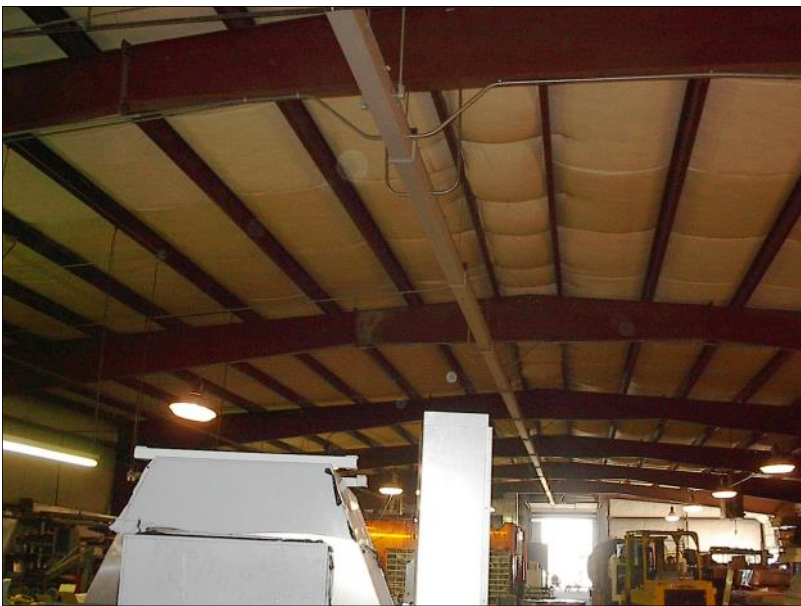
Inside ceiling view End to end showing insulation and steel beam construction.
